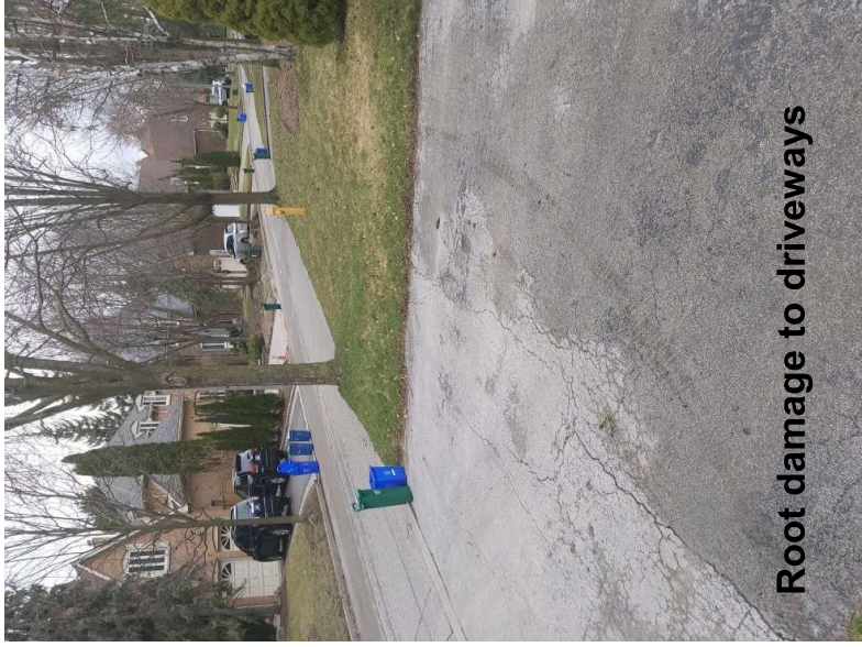
Cracked or damaged sidewalks
