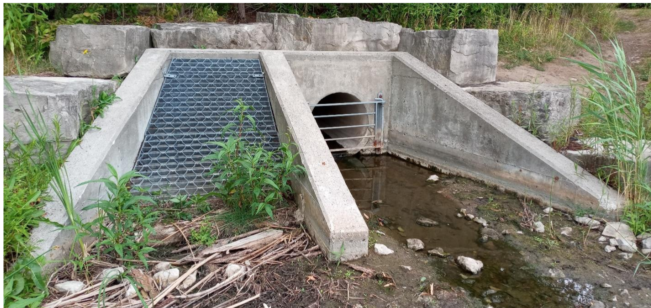
Lake Outflow Grate
