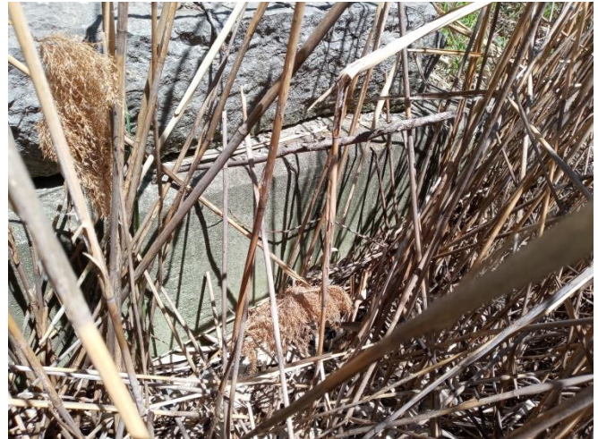
Blocked outlet from Swan Club Separator to Swan Lake (May 2021)
