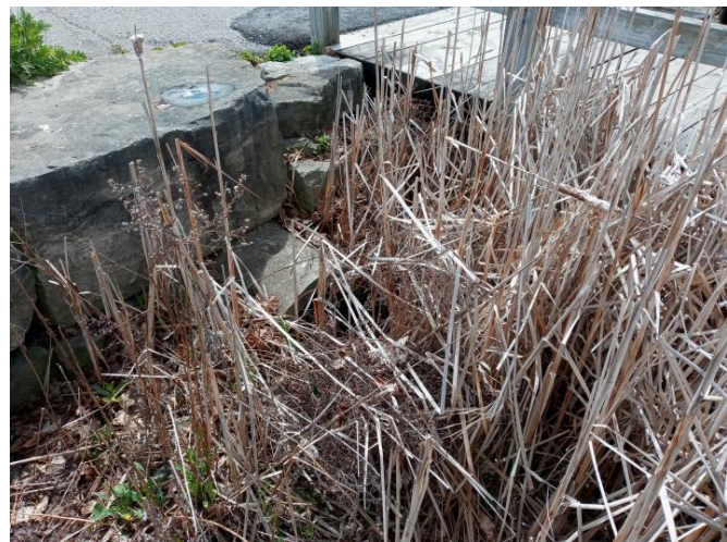
Outlet from Traffic Circle Separator to Swan Lake. Appears functional though somewhat overgrown.
