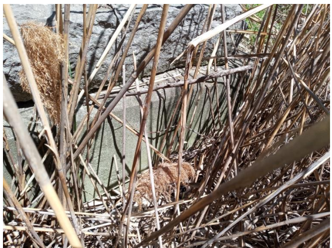
Clogged Inlet to Swan Lake (May 14, 2021)
