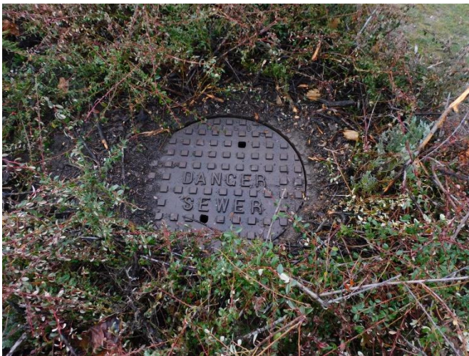
Oil/Grit Separator Uncovered December 2020
