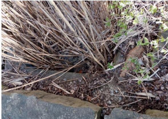
Blocked Splitter Channel – East Pond April 2021
